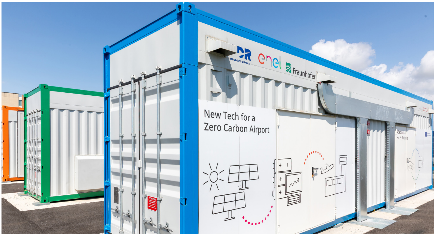
▲ Image 3.6 Enel's Pioneer BESS site in Rome
