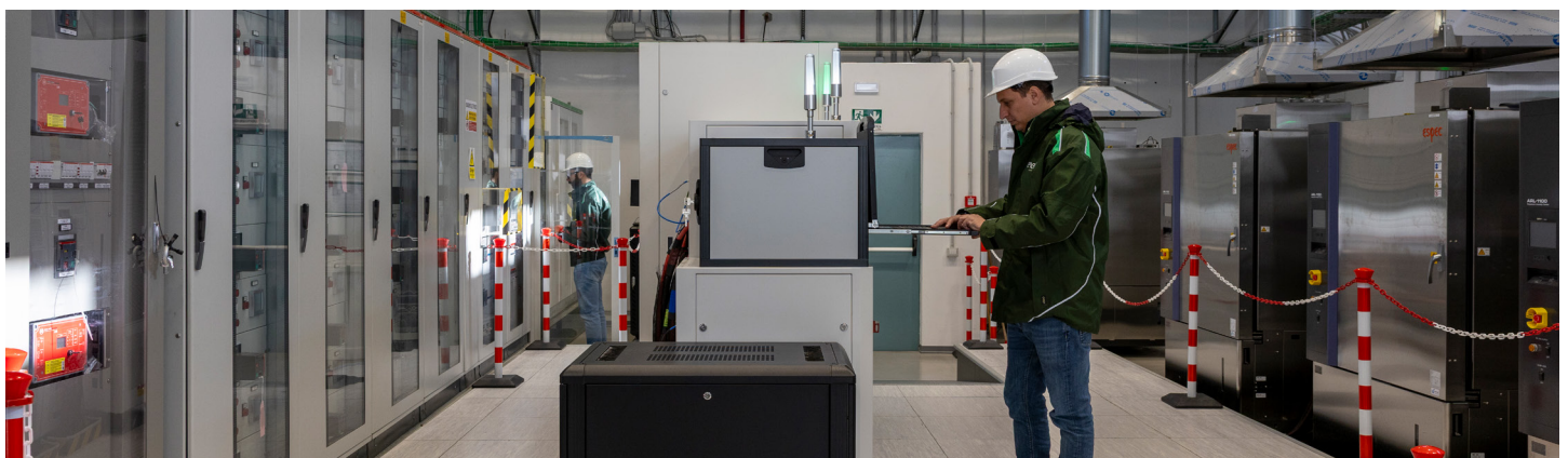
▲ Image 3.5 Storage testing facility at the Enel Catania Innovation Lab
