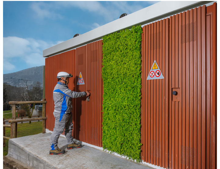
▲ Image 3.13 Enel's new secondary substation
