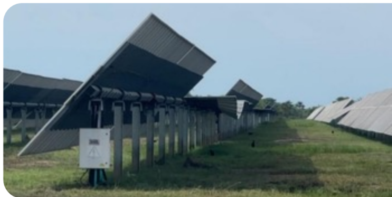
▲ Image 2.9 Impact of extreme wind on the “El Paso” solar plant
